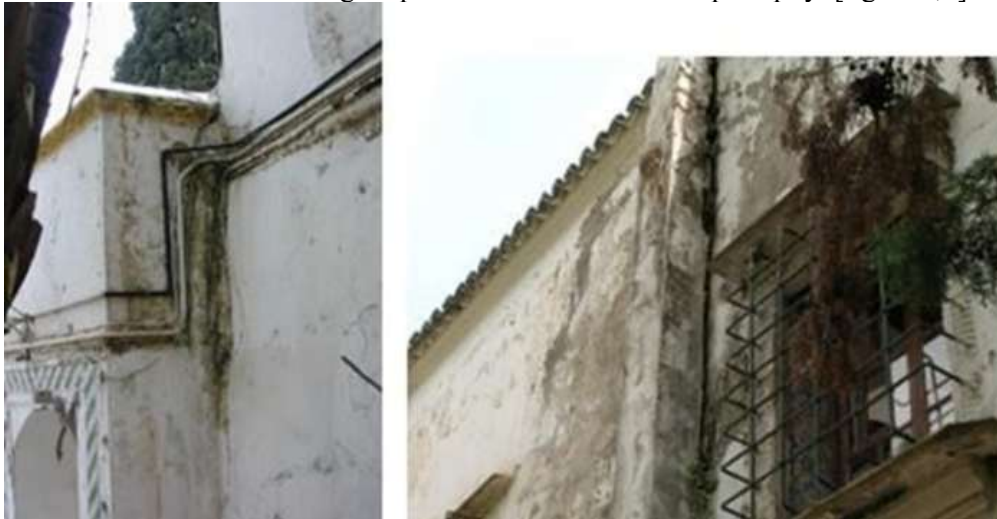
Figure 2: The Degradation Of A Façade Due To The Rupture Of The Rainwater Drainage System (National Museum Of Bardo).
