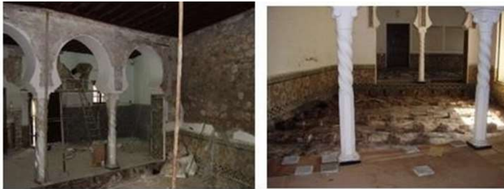
Figure 3: (Left) Mold in Interior Spaces Affecting the Tiles + Degradation of The Coatings. (Right) Stripping of The Damaged Coatings (National Museum of Bardo).
