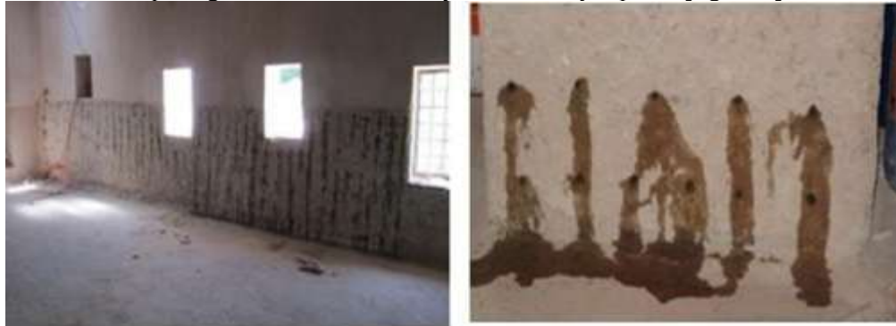
Figure 6: Drilling And Injection of a Waterproofing Solution (Prehistory Room) (National Museum of Bardo)
