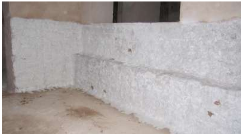
Figure 7: Moisture Treatment Wall: Anti-Salt Barriers) (National Museum of Bardo)
