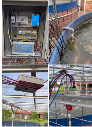
Figure 3. Field Implementation of HMI and PLC
