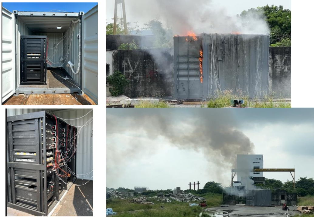
Fig. 4 Combustion experiment of a 10-foot energy storage cabinet
